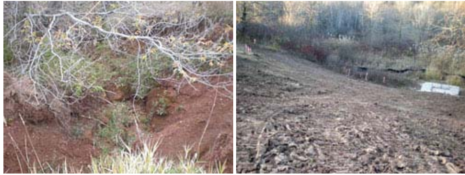
Embankment before and after construction. Photos courtesy of Glacierland R C & D
