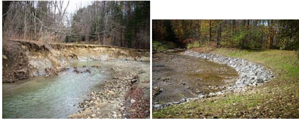
Streambank before and after construction. Photos courtesy of Erie County Soil and Water Conservation District
