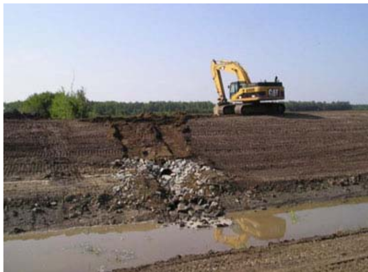
Photos: Judicial Ditch 28 before and during construction of a 2-stage ditch Bostic and Zippel Creeks Watershed Assessment Project Grantee: Lake of the Woods Soil and Water Conservation District, Minnesota
