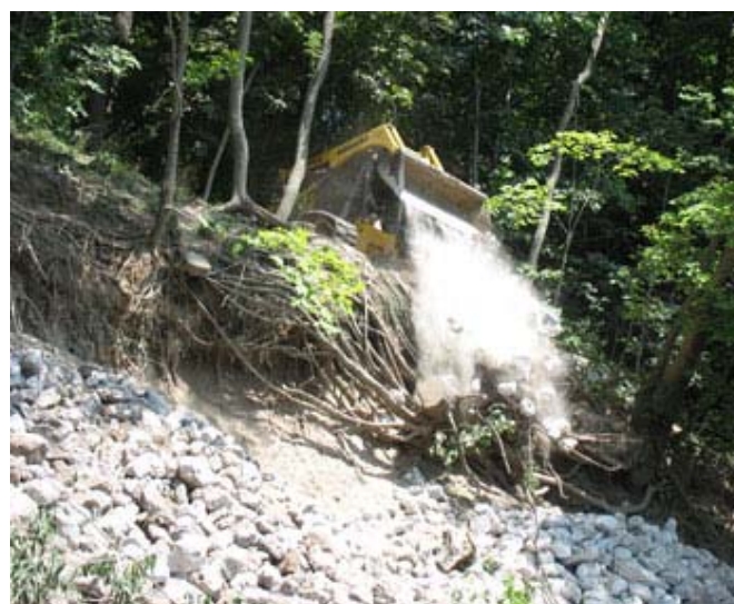
Photo: Installation of the Rock Toe Project #150802: St. Joseph River Bank Stabilization Project Grantee: Sisters of the Holy Cross, Indiana
